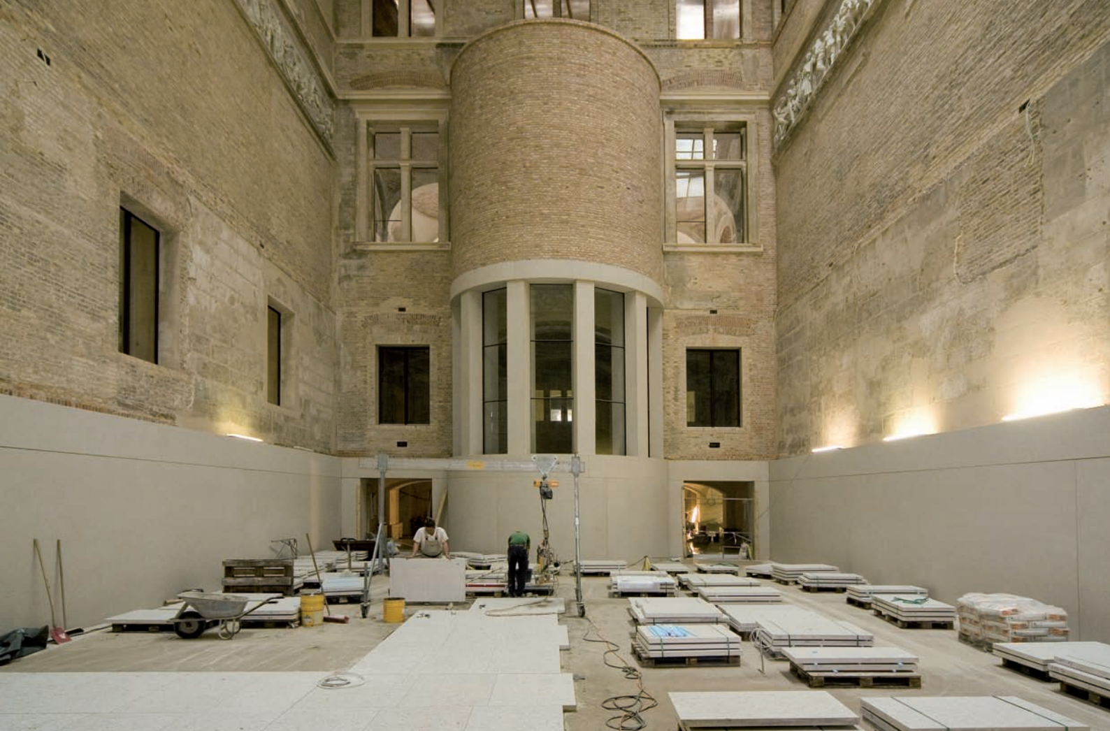
Laying the floor slabs in the Greek Courtyard with its distinctive apse
